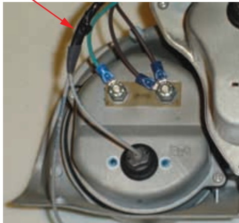
Water Temperature Gauge Connections
